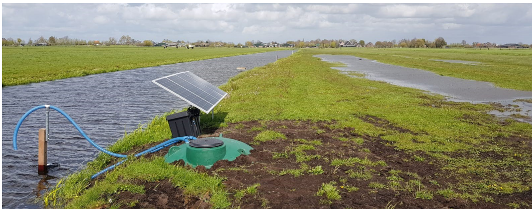
Foto: Waterinfiltratiesysteem (WIS)
